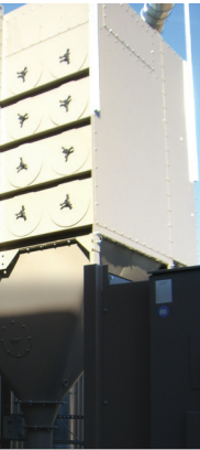
dust collector protected enclosures with a
